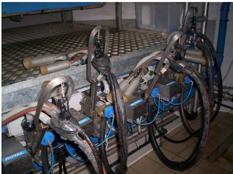
Figure 1. The innovative flow-based ACR installed on the milking parlour of the experimental farm of the University of Milan
