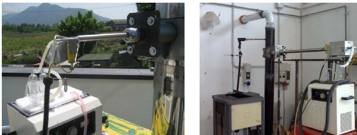
Figure 2. Ministack probe on boiler chimney (left) and pellet stove (right).
