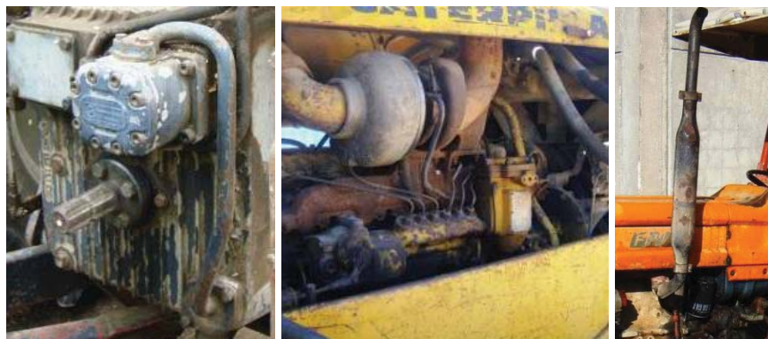
Figure 11. Left: transmission shank without any protective shield or shelter covering the terminal outlet of the PTO. Centre: the transmission belt of the fan and large part of the engine compartment do not have protections against accidental contacts on both sides. Right: a pipe for exhaust gas without protection against accidental contacts. It is located very close to the access to the tractor cab
